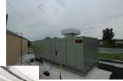
High Efficiency HVAC
